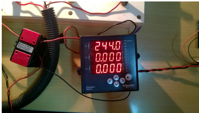
Figure 11.11: Single Phase Voltage Output on Energy Meter
