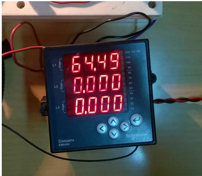
Figure 11.13: Single phase active power output in energy meter
