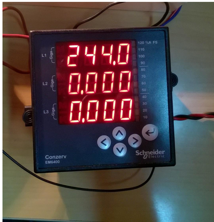
Figure 11.11: Single phase voltage output in energy meter
